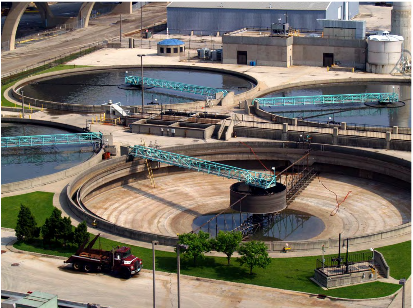
The construction of these large primary clarifiers at the water reclamation facilities is funded through the capital budget, but the maintenance is funded through the O&M budget.
