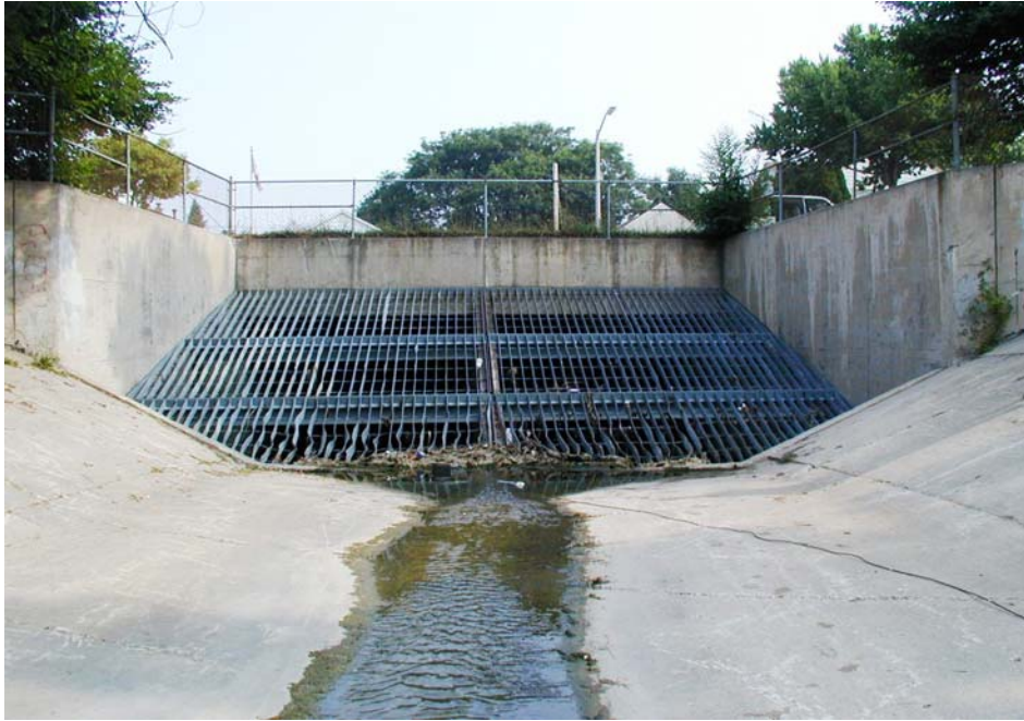
Figure 3. Honey Creek entering underground conduit at 81 st Street and Arthur Avenue (north end of McCarty Park).
