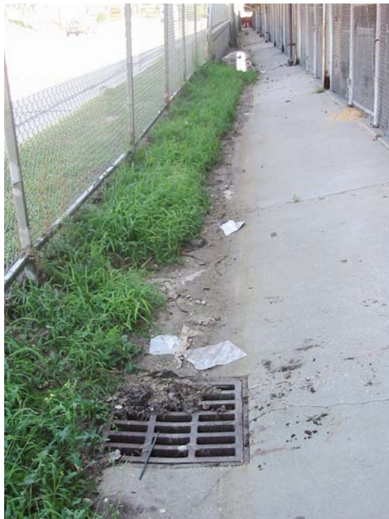
Figure 18. State Fair Storm Sewer Grate
