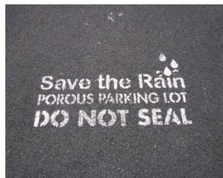
Signage and other displays such as pavement markings can help ensure proper O&M takes place
